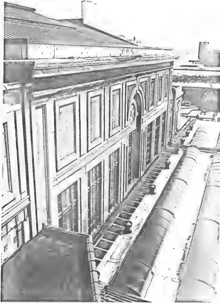
Western facade of terminal, viewed from roof of train concourse. Note large gap in section of copper cornice above arch.
